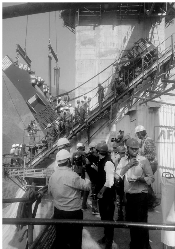
Engineers perform puja on Judda side of the world's tallest railway bridge in Reasi district, connecting Bakal and Kauri areas to begin the last phase of work of connecting the huge arch 1,178 ft above river Chenab on under-construction Jammu-Srinagar railway line which will connect Kashmir to Kanyakumari, in Jammu on Sunday. — PTI
